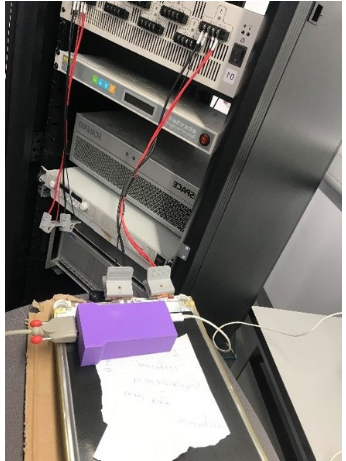
Fig. 2 Placement of the sensors on the surface of the cell for directly measuring the magnetic field for online magnetic field monitoring while charging.
